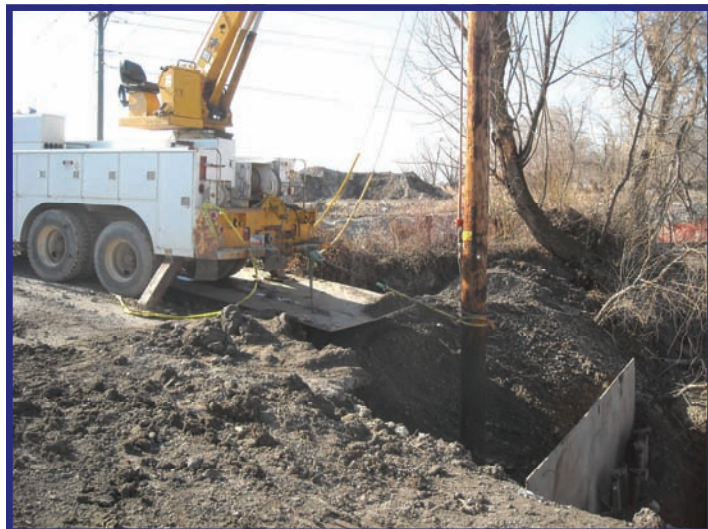
Electrical utility truck holding an existing electrical pole next to COP's 25' deep utility excavation (Photo by Jasen Bennie)
