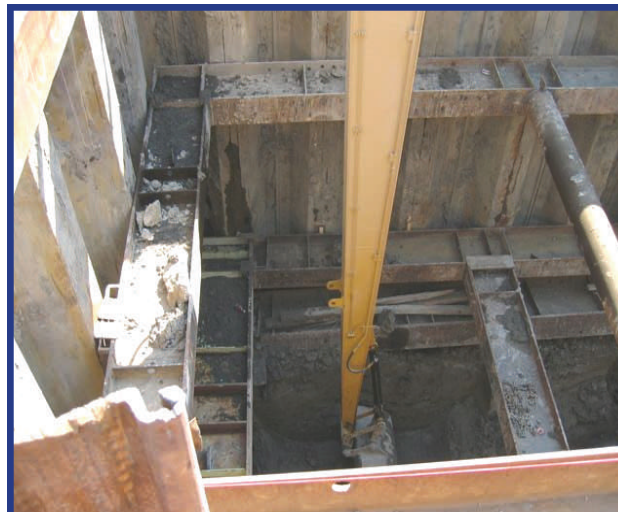
Long stick excavator digging out sheet pile cell (Photo by Jasen Bennie)
