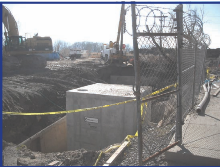
Precast meter vault (Photo by Jasen Bennie)
