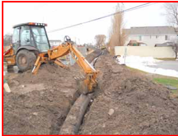
The HDPE had to be encased in flowfill along the canal; the pipe had to be held down to keep it from floating.
