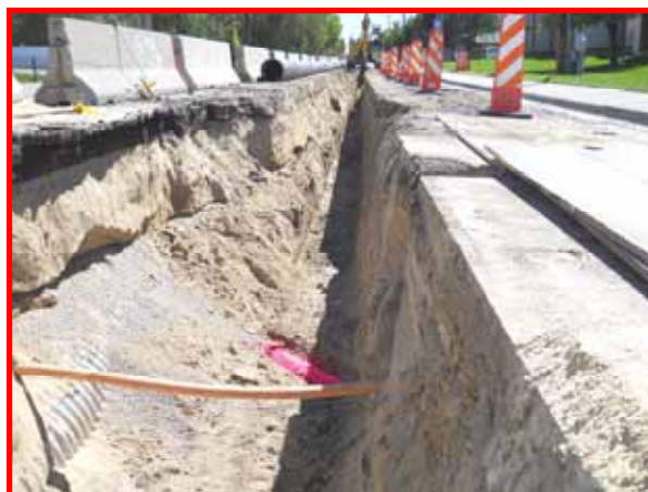
To avoid road closures, the work area was barricaded off to accommodate traffic flow.
