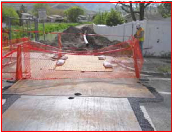
Limited space along the canal added to the difficulty of installing this pipe.
