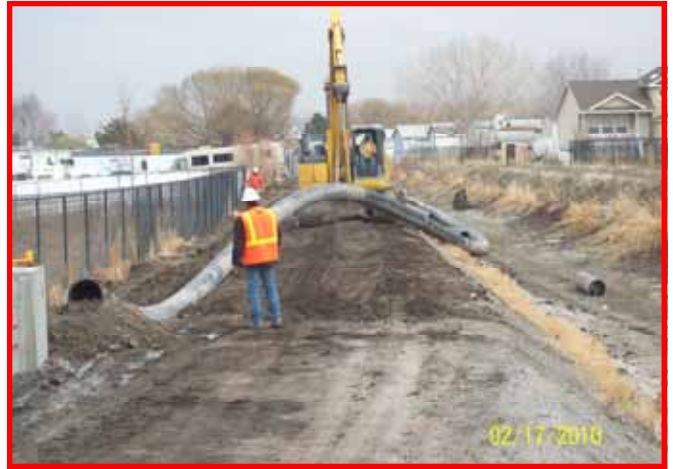
Along the canal long sections of pipe were installed after all of the trench was excavated.
