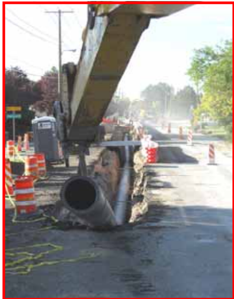
In the road section long trenches would be dug to expose all utilities; the pipe was threaded through to install it.
