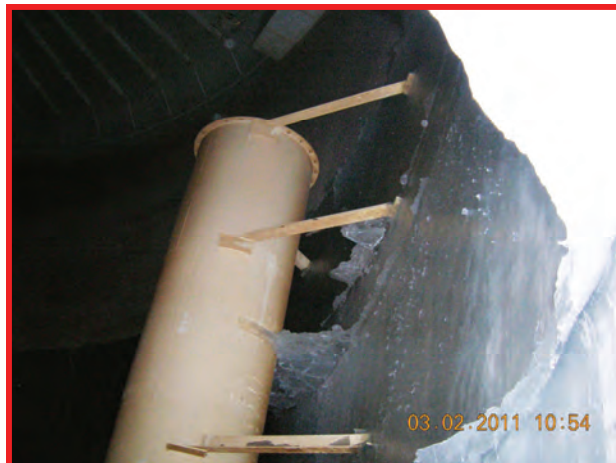
Inlet pipe inside clearwell with ice build-up on walls.
