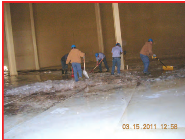
City crew breaking up 14 inches of ice on floors before project could begin.
