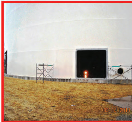
10' x 10' access opening cut into wall of clearwell. Photo by Joe Allen
