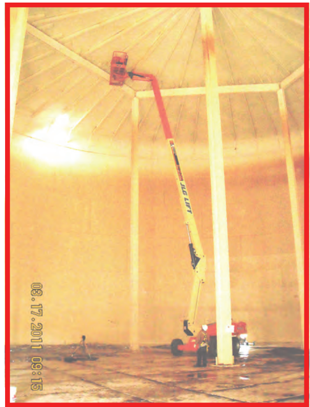
Welding bar onto the rafters used to support the baffle. Photo by Joe Allen
