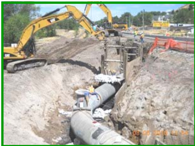
60" mainline pipe on Hwy 89 with area ready for concrete manway structure. Photo by Jade Lee
