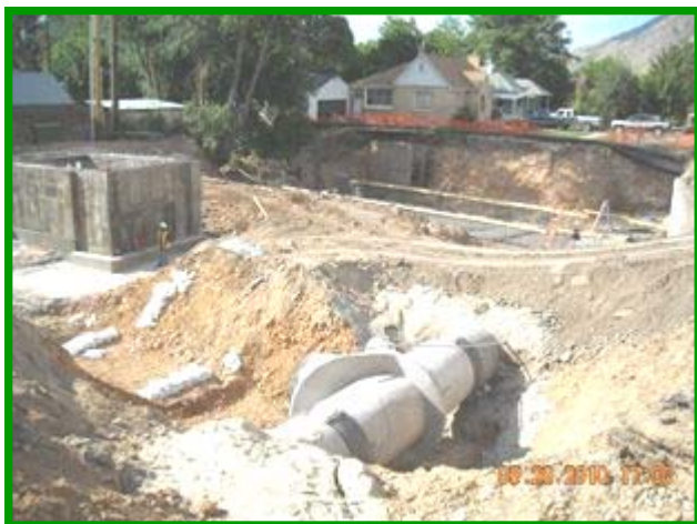
View of Hobble Creek work area — deep wet well, box culvert, and 60" mainline tee. Photo by Doug Teller
