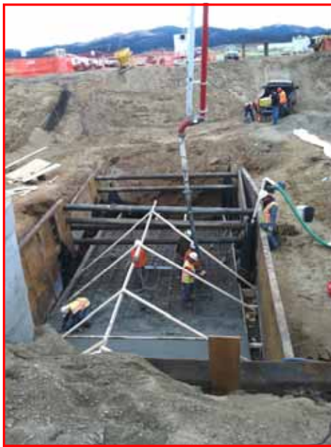
COP concrete crew pouring deep slab foundations for Lift Station #2. Photo by Doug Teller
