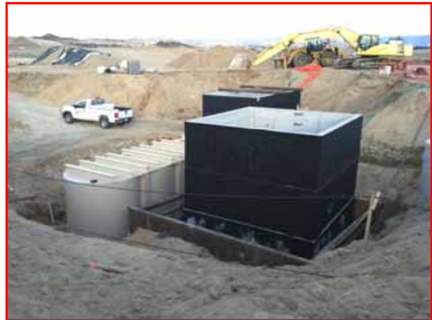
Lift Station #2 wet well, Pig Launcher Vault, and steel lift station structures. Photo by Doug Teller
