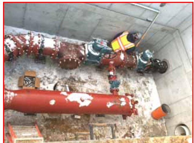
Mechanical piping inside Pig Launcher Vault. Photo by Doug Teller
