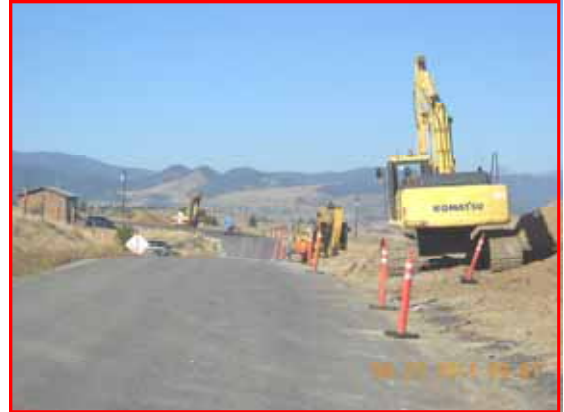
Crews #1 & #2 approaching the connection point of the two halves of the job. Photo by Greg Schied
