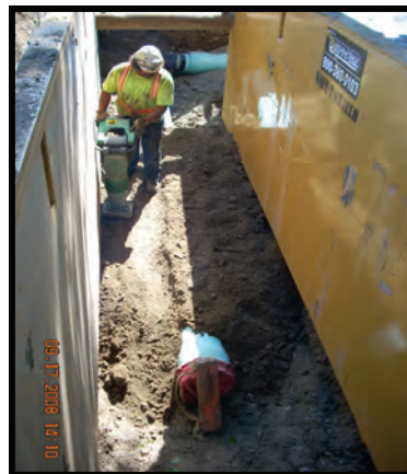
Photos above: Waterline installation at the north end of Shiloh, near Poly Drive.
