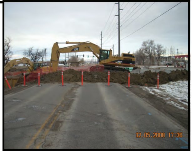
The crew crossing Shiloh Road with deep sewer, using COP's Cat 365 excavator. (Photo by Larry Brunmeier)
