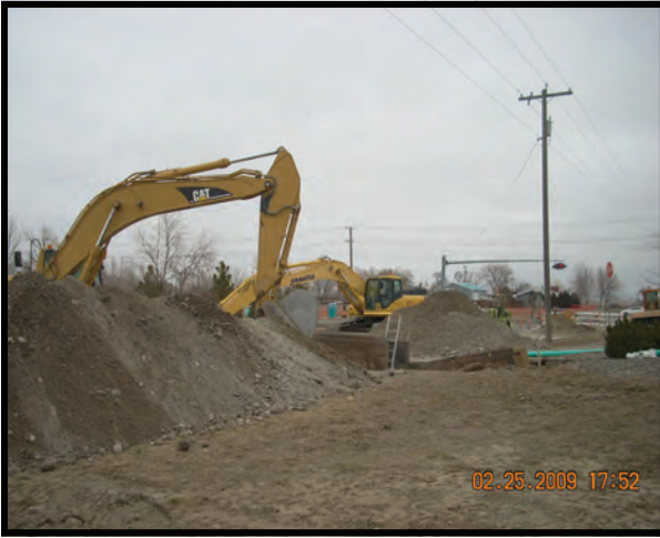
The crew completing deep sewer main and service at the Hesper Road intersection. (Photo by Larry Brunmeier)
